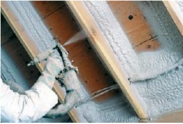
Photo of SPF being applied to wood deck using picture framing technique. Spraying foam onto a metal panel surface would be done in the same fashion.
