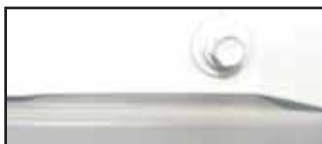
Minimal corrosion is detected along cut end of panel with Edge-Rust Inhibitor application.
